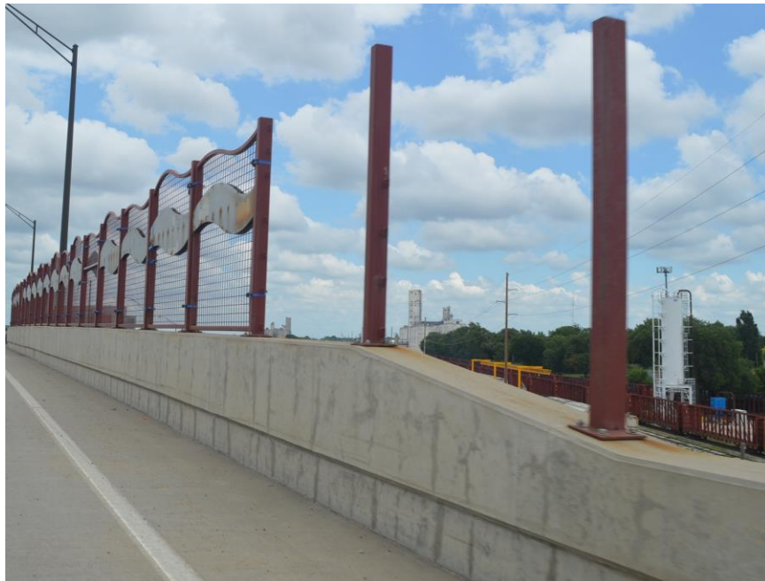
Figure 49. Aesthetic Design Missing Panels
